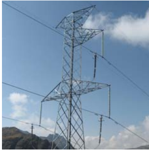
Transmission line arresters
